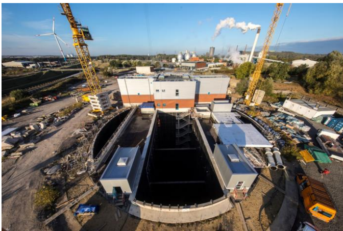
The construction site of the Bottrop pumping station on the grounds of the Bottrop sewage treatment plant in 2016.
